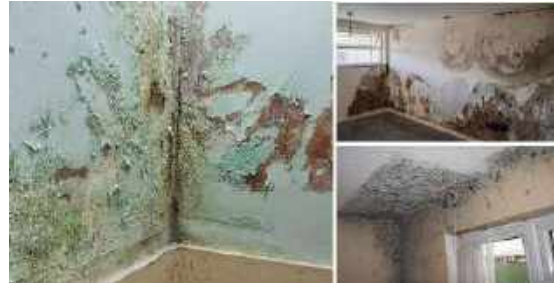
Figure 1 Dampness in masonry
